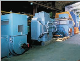
Storage of critical spare motors
