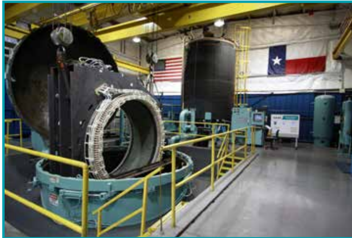
IPS provides ABB authorized "global VPI" rewinds up to 13.8 kV. The IPS Houston 14' x 17' VPI tank is the largest in the United States, and it is located in a dedicated winding clean room environment.
