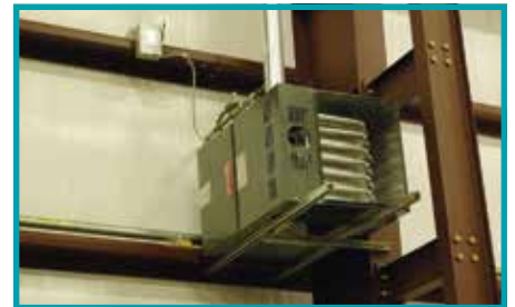
Heaters and dehumidifiers maintain relative humidity at 50% or lower, preventing condensation and meeting IEEE specifications
