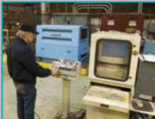
Load testing to 1,500 HP and 13.2 kV / 500 VDC
