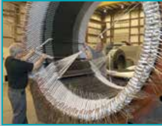
IntegraCoil™ 15 kV stator rewind
