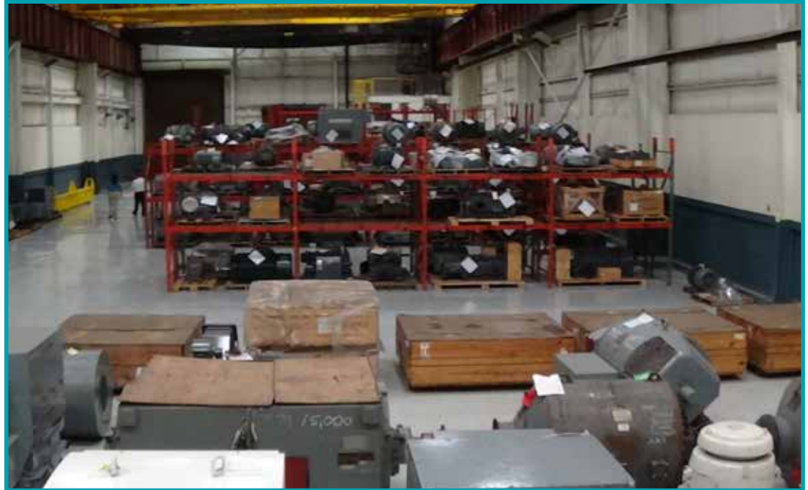
The IPS Cleveland Service Center has extensive experience in the professional storage and management of small, large and extra-large motors and generators
