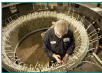
In-shop motor and generator repair
