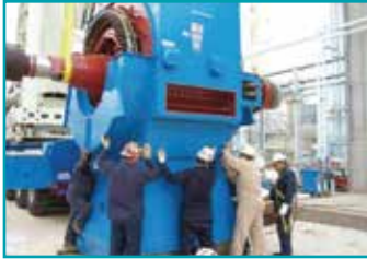
Extensive on-site field services
