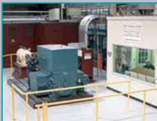
Testing up to 37,500 HP and 15 kV / 700 VDC
