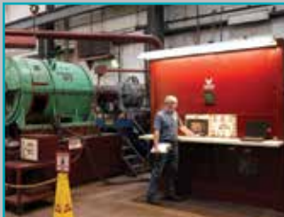
Load testing to 1,500 HP and 13,800 VAC / 750 VDC
