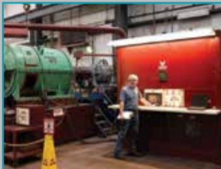
Load testing to 1,500 HP and 13,800 VAC / 750 VDC
