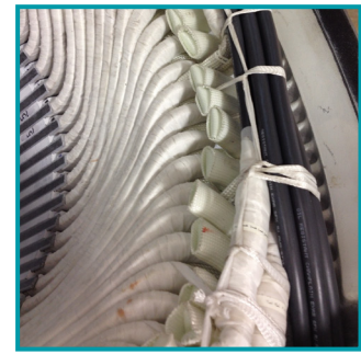
Low cost "Stub" connections & limited blocking, bracing & lashing
