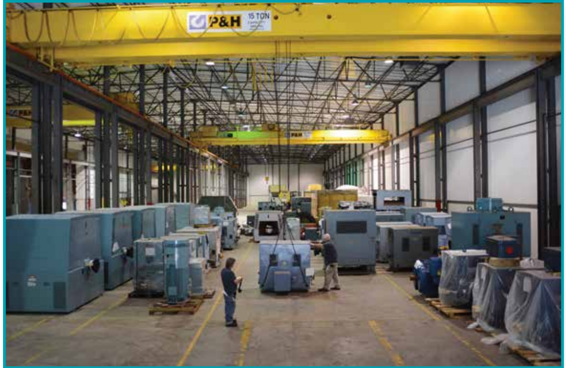
The IPS Rock Hill Service Center has extensive experience in the professional storage and management of process critical, small, large and extra-large motors and generators
