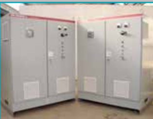
Custom Control Panels
