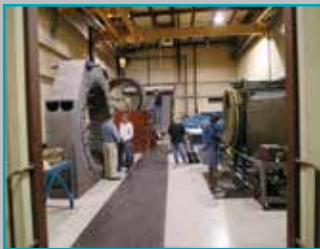
Dedicated winding clean room with 12' VPI tank
