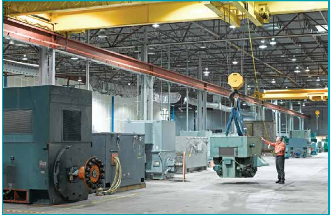
The IPS Shreveport Service Center has extensive experience in the professional storage and management of process critical, small, large and extra-large motors and generators
