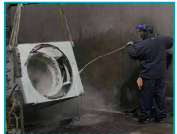
IPS reconditioned both motors, including the safe removal of contamination and debris, in order to prevent future winding failures and costly motor rewinds.
