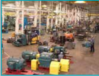
Service center has 64,000 sq. ft. and 40-ton lifting capacity
