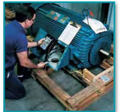
Coils are Meggered quarterly (or to customer specification)
