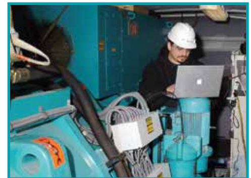
IPS technicians provide complete inspections of mechanical components before warranties end, to minimize repair and replacement costs
