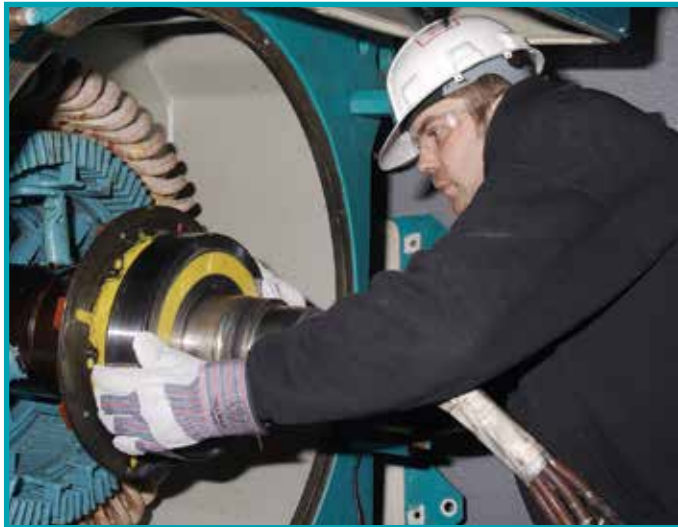
IPS offers a full range of predictive and preventive maintenance services, including wind generator bearing change outs and upgrades
