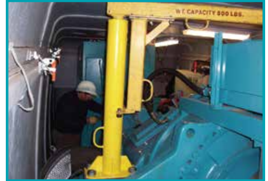
IPS technicians have spent years working up-tower, refining the technologies needed to handle and machine heavyweight components inside the nacelle
