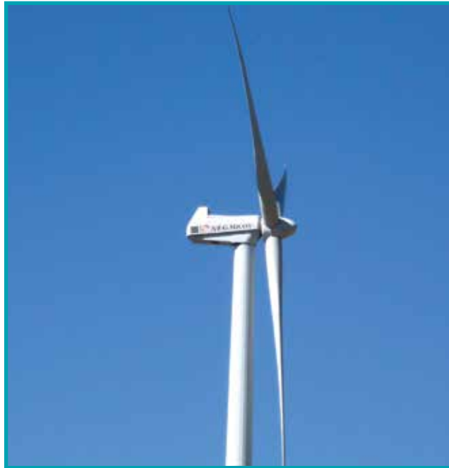
Our dedicated up-tower and in-shop technicians service NEG Micon turbines coast to coast
