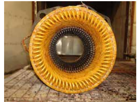
After: PowerSeal windings after cleaning are like new
