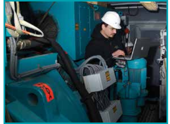
IPS Litchfield's field service team provides on-site commissioning, repair, preventive and predictive maintenance services for your motors and generators
