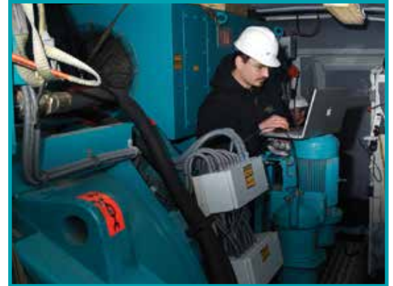
IPS Portland's field service team provides on-site commissioning, repair, preventive and predictive maintenance services for your motors and generators
