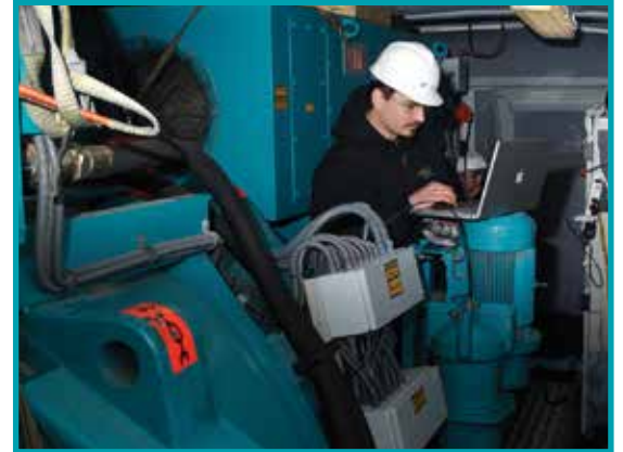
IPS Cleveland's field service team provides on-site commissioning, repair, preventive and predictive maintenance services for your motors and generators
