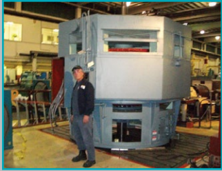
Testing to 750 kVA - 4,160 V, 500 VDC
