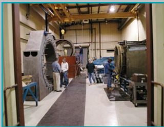
Dedicated winding clean room with 12' VPI tank
