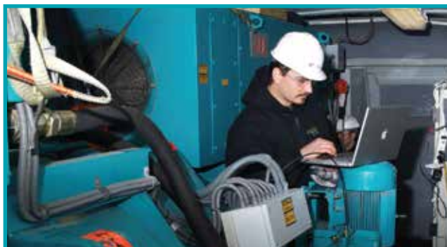
Our up-tower technicians provide predictive and preventive maintenance, diagnostic testing and pre end-of-warranty inspections
